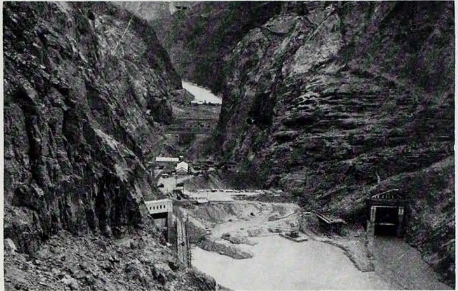
Work begins in Black Canyon of the Colorado River: at lower right is the mouth of a diversion tunnel.
