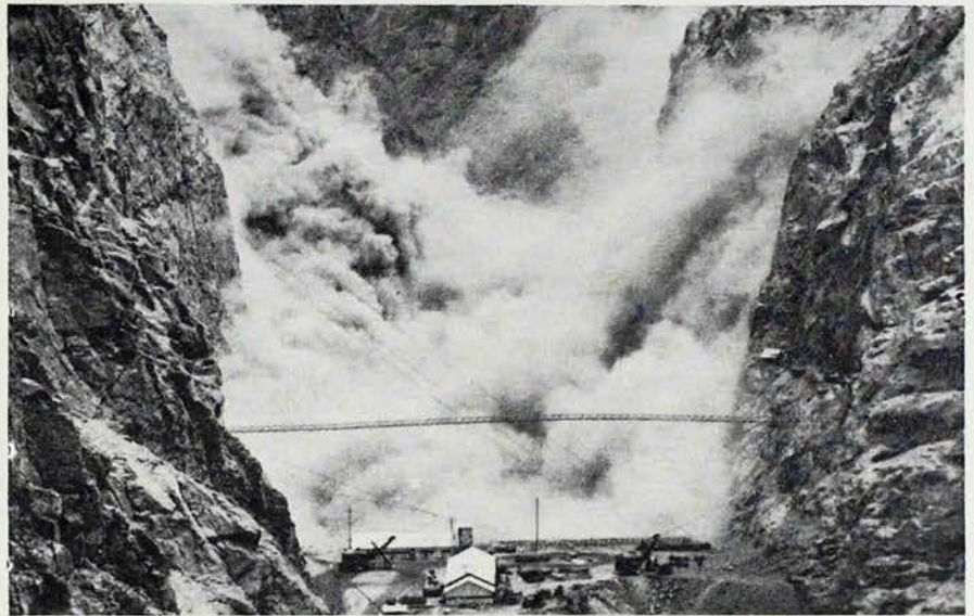
Last big blast to shape the face of the canyon to fit concrete wall of Boulder Dam.
